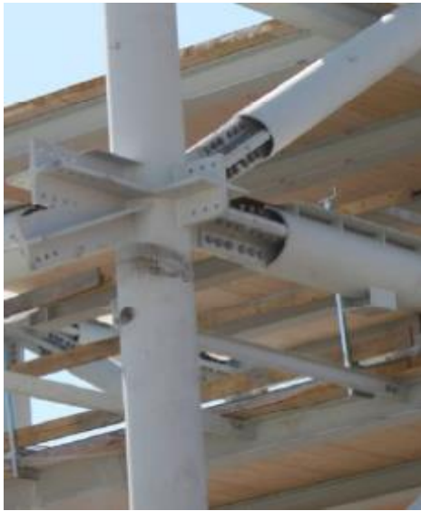
Figure 2.7: Example of a hollow section joint materialised with stiffeners and bolting (EXPO 2015 Construction).
