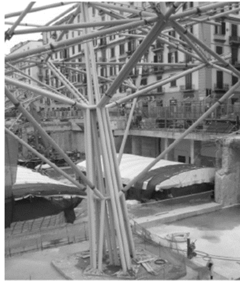
Figure 2.8: Steelwork made with CHS elements processed by laser cutting technique (Piazza Garibaldi roofing in Naples, Italy).
